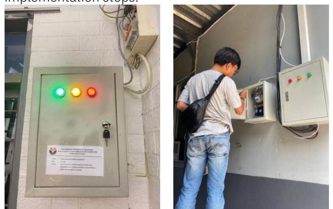
Figure 8. Power Meter Implementation
